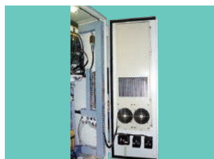
盤内エアコン Air conditioner in control box
