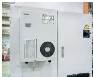
盤内エアコン Air conditioner in control box
